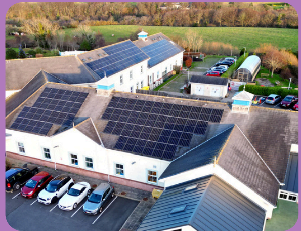
We've taken important steps towards improving sustainability and saving money, with the installation of new solar panels
